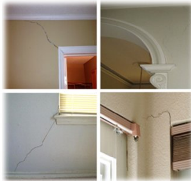
Fig.1: Cracks that appear in walls around architectural openings like doors and windows over time.[3],[4],[5],[6]
